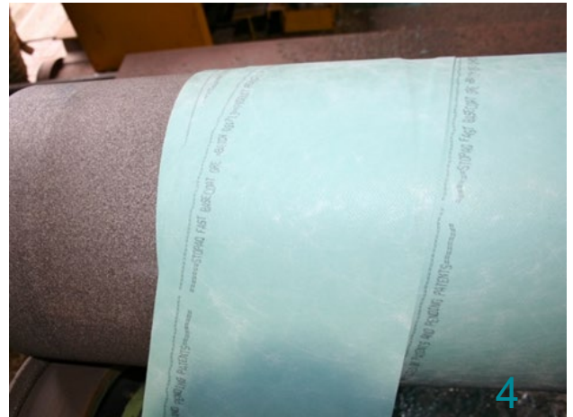
Continue the entire area has been wrapped with FAST Basecoat. Conduct holiday test at 10kV with a brush probe.
