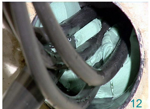
Lift the cables and apply the 2100 Aquastop with a suitable injection tool around the cables.
