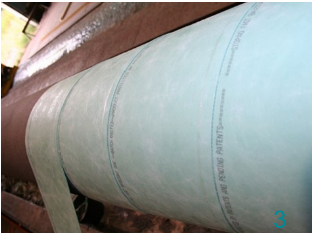
The overlap can be adjusted by changing the travel speed of the FAST Basecoat Wrapping Device. New rolls shall be installed with a minimum circumferential overlap of 50mm.
